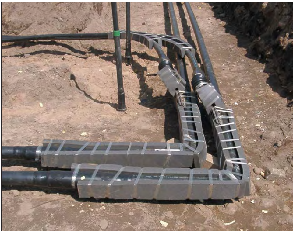
Figure 5. Local heating network with distribution pipeline (rigid pre-insulated bonded pipe) / house connection pipeline (flexible steel pipe)
